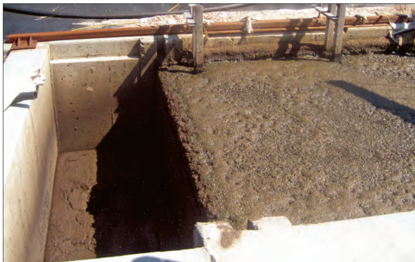
In a two-stage anaerobic manure digestion system the process is separated into distinct portions, mirroring the biological process. High solids waste are placed in a concrete bay where water is passed through, effectively leaching out organics that are later converted into methane gas.
